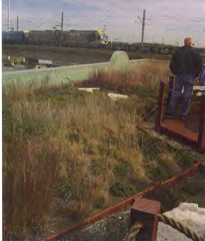
The roof at the Green Institute in Minneapolis collects and filters rainwater on its roof.
