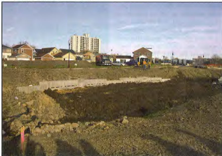
This stormwater control system is under construction at the Heritage Park Development in Minneapolis.
