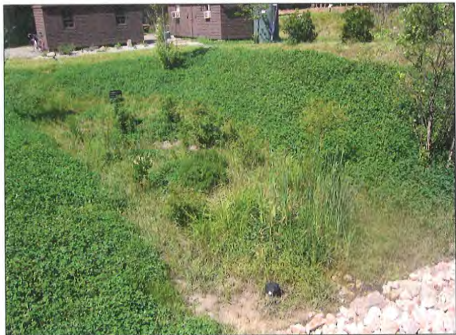
A gravel wetland was constructed at the UNH Stormwater Center. The photograph is courtesy of the UNH.
