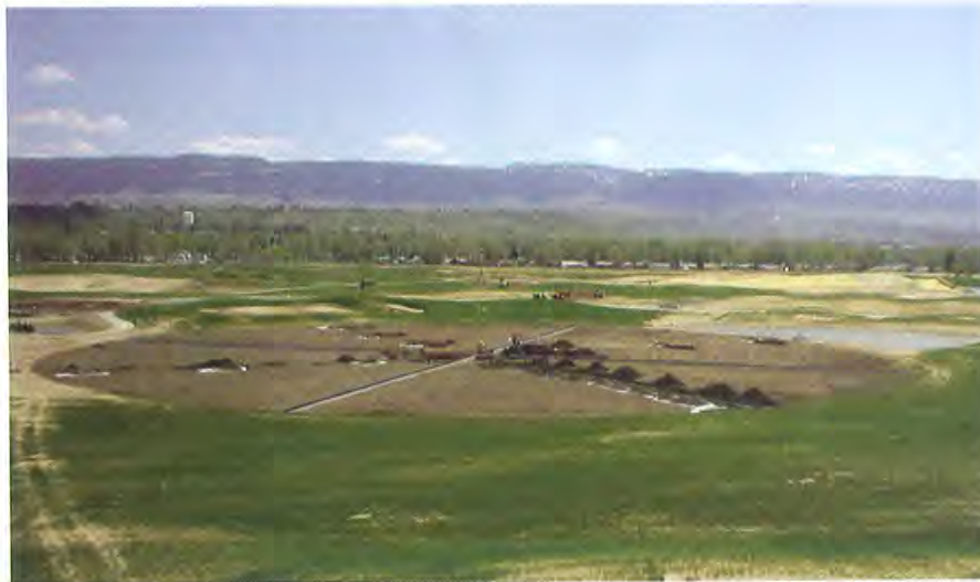
Subsurface flow constructed wetland near completion at former BP site. The wetland is being covered with a tan mulch layer to ensure cold-weather operation during the winter months.
