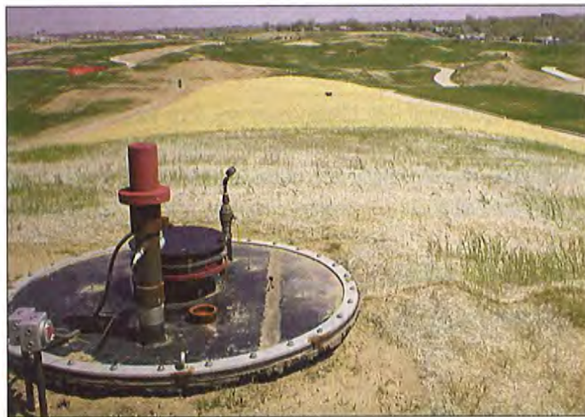
The treatment system had to handle up to 3 MGD of gasoline-contaminated groundwater, blend into the middle of a premier golf course, and operate for over a century.
